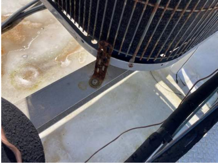
Figure 23 corroding AC unit bracket typical
