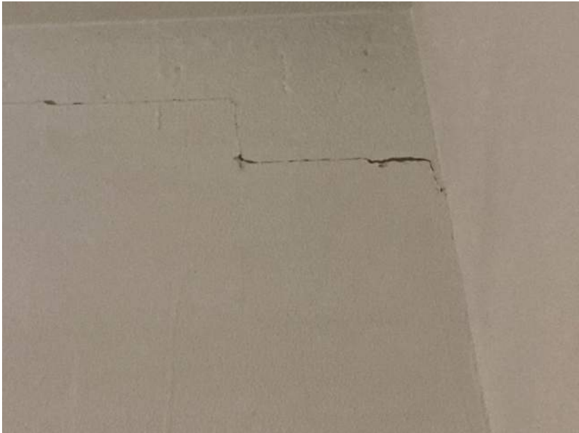
Figure 18 One location of Stairstepping
