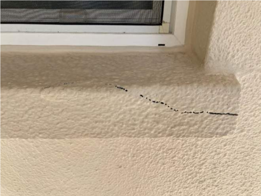
Figure 17 One location of Window Sill cracking
