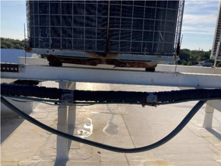
Figure 22 corroding AC unit typical
